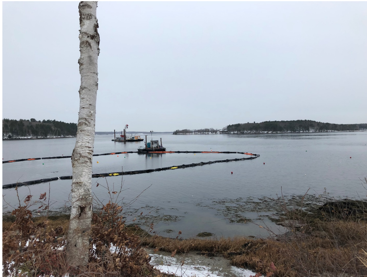
East side diver burial in channel. Turbidity barrier is in initial installation stage with diver working just outside of barrier. Work barge with concrete mattresses in the background.
